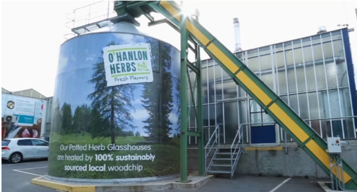
O'Hanlon Herbs woodchip conveyor and silo
